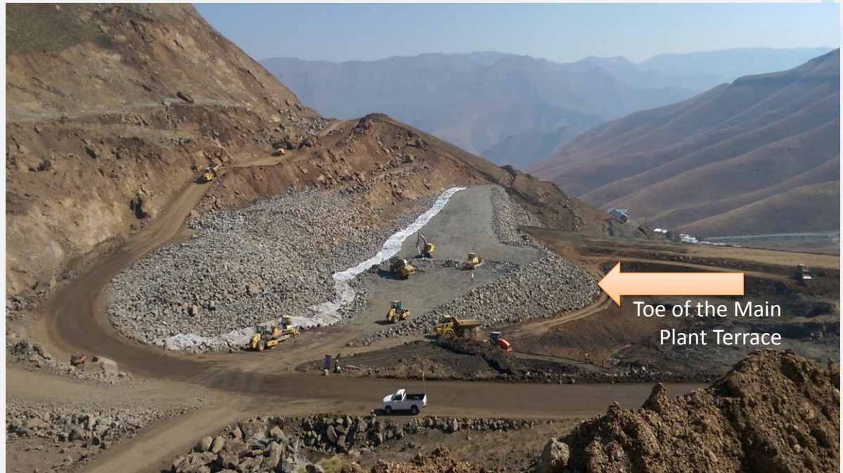
Main plant terrace May 2015
