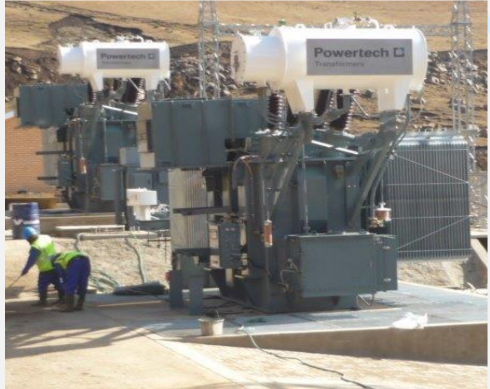
Substation with transformers installed May 2015
